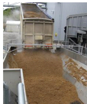
The plant utilises draff which is a by-product of whisky production. This comes from 17 different distilleries and is mixed 50/50 with wood chips.
