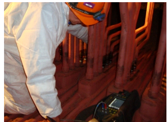
The combustion system is examined and improved.
