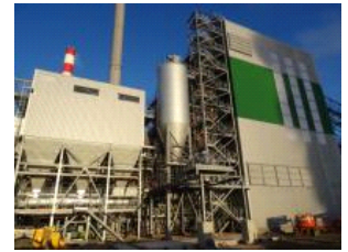
The Biolacq Energies project, in Lacq, is a biomass-fired CHP plant of 54 MW, that utilises forestry wood, and clean, uncontaminated residues from wood processing.
