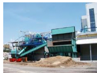
Fuel conveyer line.
