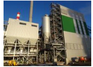
The Biolaq Energies project, in Lacq, is a biomass-fired CHP plant of 54 MW, that utilises forestry wood, and clean, uncontaminated residues from wood processing.
