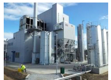
Roth's CoRDe CHP Plant, Scotland.
