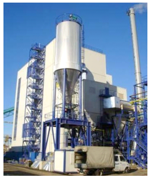
FunderMax reduced the NO x emissions approx. 80% by using the AET SNCR DeNO x System.
