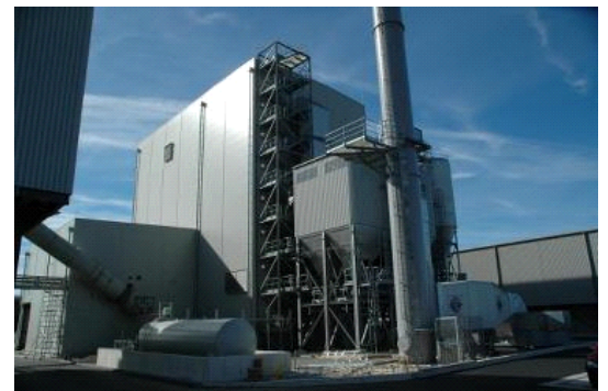
The Western Wood biomass power plant has a 48 MWth AET Biomass Boiler with the latest AET Combustion System , - which fulfills stringent NOx emission criteria without SNCR. Power production is 15 MWe.
