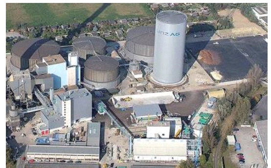
18% of all district heating for Linz, the third-largest city of Austria, is served by a biomass-fired combined heat and power (CHP) plant.
