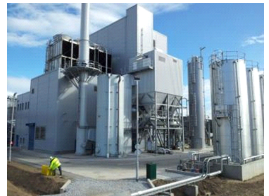
Helius CoRDe Ltd is a biomass-fired cogeneration plant in Scotland fuelled with a whisky by-product and clean wood. The plant was commissioned in 2013.
