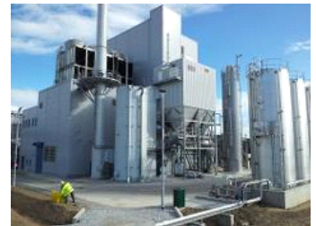
The Rothes CoRDe cogeneration plant produces heat and power.
